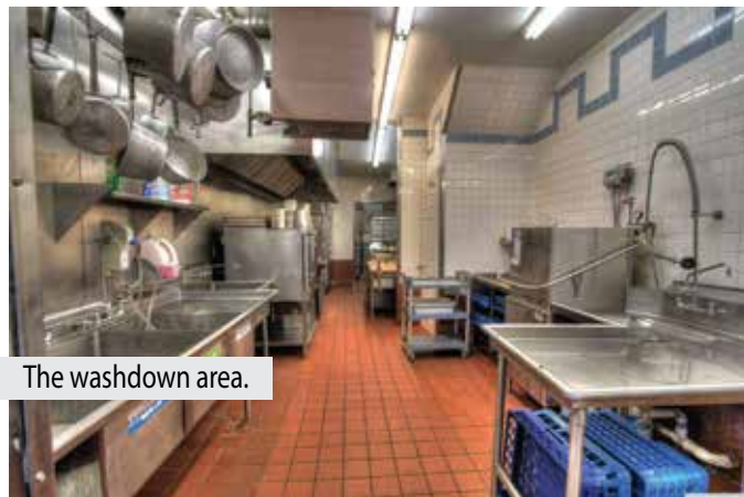
The complete kitchen with walk in freezer and work area.
