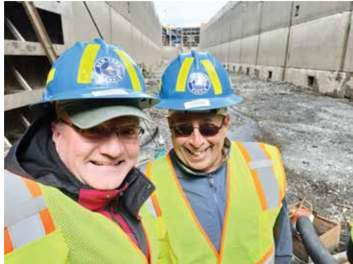
The author (left) with Larry Ascenzi of Lock One Marina and Shipyard, during a recent inspection tour of Lock C-2 near Mechanicville. The Canal Corporation periodically drains certain locks in order to completely inspect and overhaul their working mechanisms during the winter. It's a 12 month operation!
