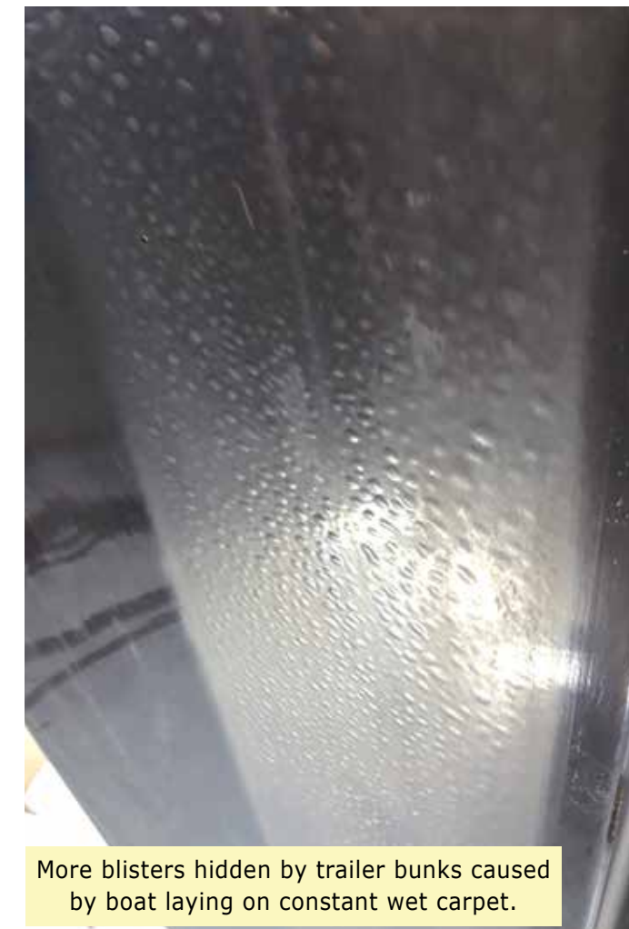
This transom should be straight across but because of cracked fiberglass in two places and rot developed.
