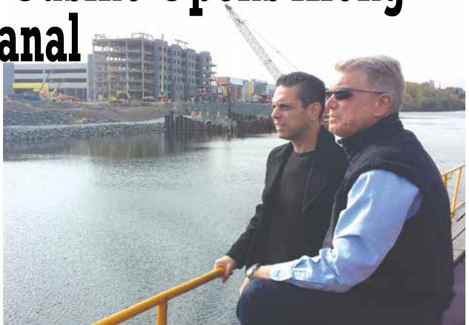
In this October 2016 photo, Canal Corporation Director Brian Stratton (right) joins Assemblyman Angelo Santabarbara aboard the Grand Erie as they survey the construction of the Rivers Casino & Resort. Unique among the state's new gaming projects, the Rivers Casino has its own protected harbor, with slips for boats up to 40 feet, and larger facilities are proposed.
